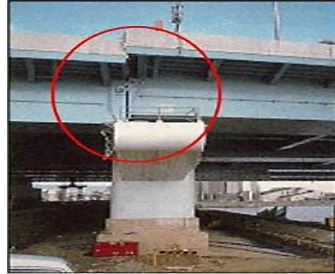
Fig. 6 Foundation instability resulting from soil liquefaction during seismic events, leading to excessive settlement and loss of lateral support for bridge substructures (Barbosa & Silva, 2007)
