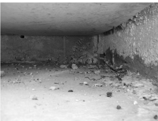
Figure 10. Concrete surfaces improperly finished.
