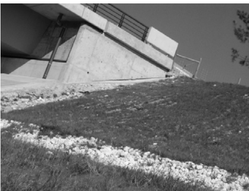
Figure 9. Cracked abutment wings.
