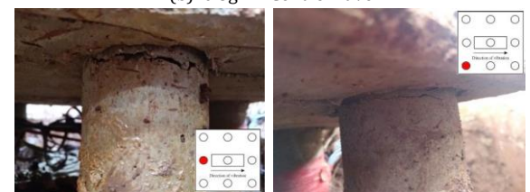
(c) The link between the piles and the piles cap has fractured (0.8g)
