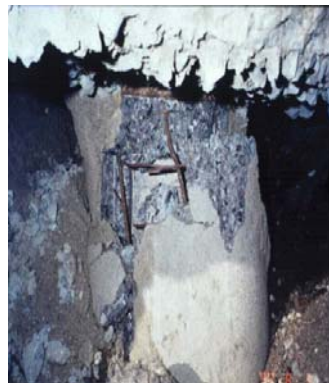
d. Damage at pile-to-pile cap connection
