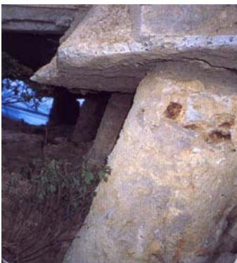
a. Inelastic lateral deformation at pile-to-pile cap interface
