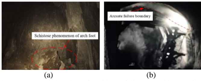
Figure 5. Actual situation of rockburst failure. a Schistose phenomenon of the arch foot; b The moment when the vault rockburst occurs
