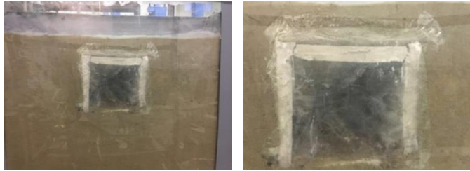
a) Cracks appearing of the metro station roof
