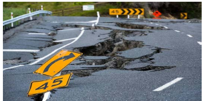
Figure 1. Earthquake damage to State Highway 1 is seen south of Kaikoura on Nov. 16.
