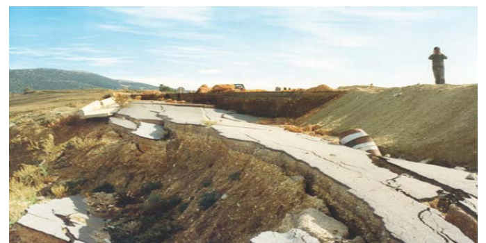
Figure 3. Significant damages to the road network. (Kozani earthquake, 1995)
