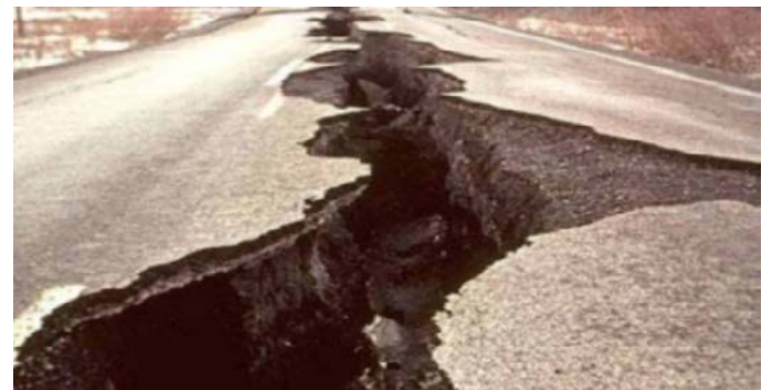
Figure 2. Roadway rupture of the provincial road (Kozani earthquake, 1995)
