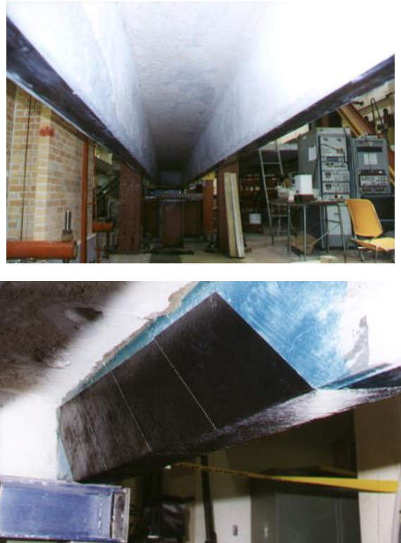
Fig. 3. HC-Type Girder after rehabilitation using CFRP strips bonded to the soffit of the web (left) and CFRP sheets bonded at the end of the web (right).
