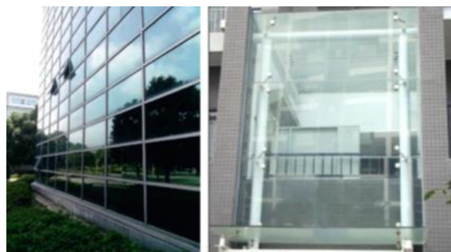
Figure 5.4 Framed glass façade (Wang et al. 2014(b)) and point-supported glass façade (Wang et al. 2014(a))
