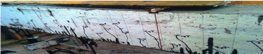
Figure 6. Failure pattern of GFRP laminated RC beam (S0 L5).
