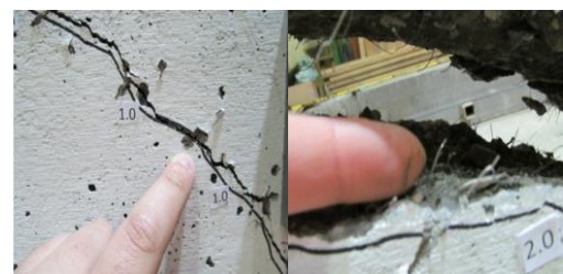
Figure 7. Other observations: (left) Control of shear crack up to 1 mm in width prior to failure in beam M15-0.5%H ; (right) observed straightening of hooked-end fibers during pullout.
