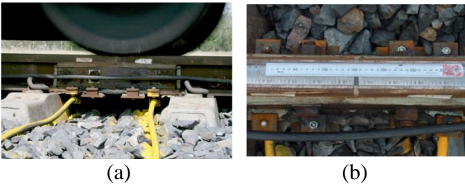
Figure 14: Field experimentation of IRJ: (a) field setup; (b) top view of IRJ.
