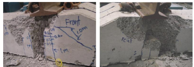
(a) Interfacial damage.
