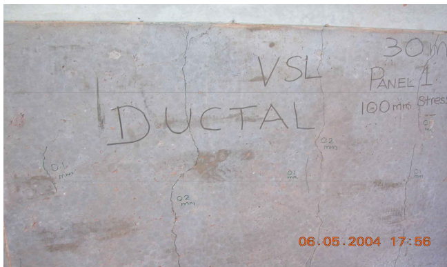
Fig. 14. Crack pattern of Ductal Panel -1
